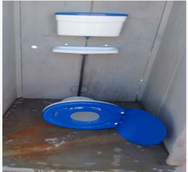
Seat in the recently installed VIP Toilets falling off in Driezik. Users are said to be falling off while seated
